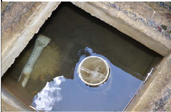
Overflow in distribution box at lower spring box location
