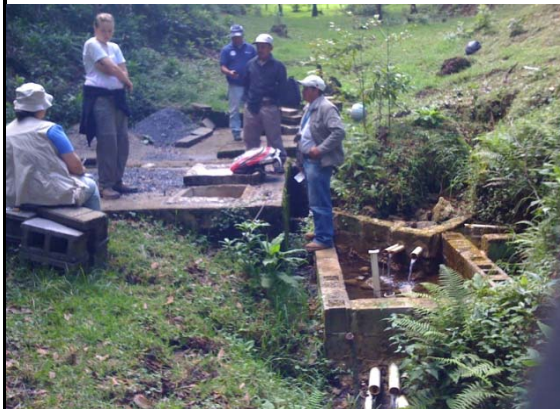
Measuring water quality at the lower spring. Open box with piping on the right is a private spring box system.
